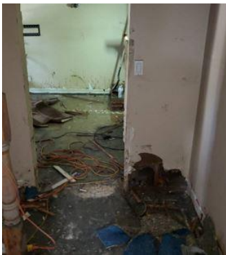
Typical FMM damages
